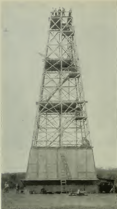
This 100-foot tower is merely a big tripod for the cameras which will get long-shots of the battle scenes in "Wings." It was built near San Antonio, Texas, where five square miles were set aside for a reproduction of the battle of St. Mihiel
