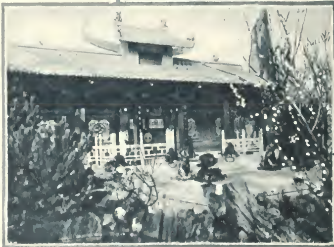
Pretty sets for " La Voile du Bonheur ," constructed at the Eclair studios. The centre picture shows the commencement of the construction.
