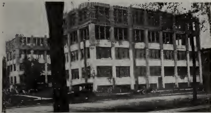
Factory of the Murray Shoe Company, London, Ont., showing new addition which will give full five stories
