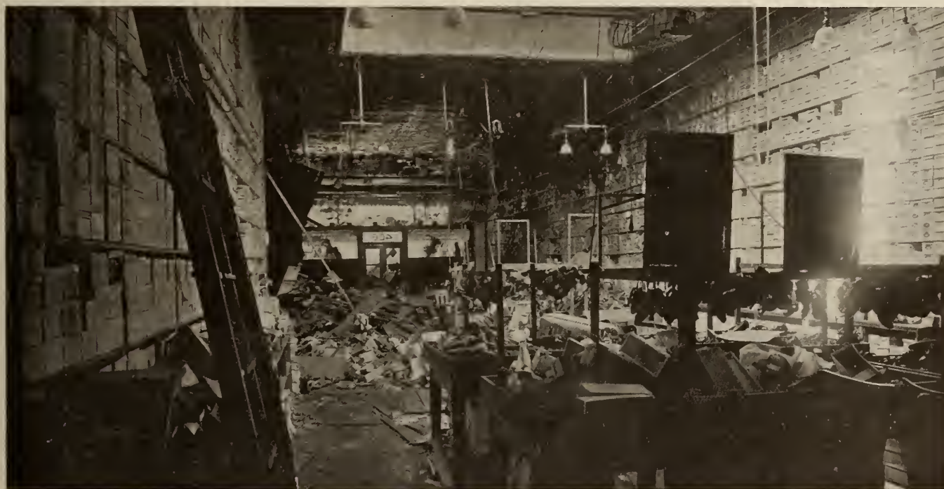
AN INTERIOR VIEW SHOWING THE DAMAGE DONE BY FIRE, WATER AND SMOKE, IN JOHNSTON'S BIG SHOE HOUSE, HASTINGS ST., VANCOUVER, ON JULY 3RD LAST. THE STORE IS NOW BEING REMODELED AND REBUILT AFTER A BIG CLEARING SALE OF THE STOCK.
