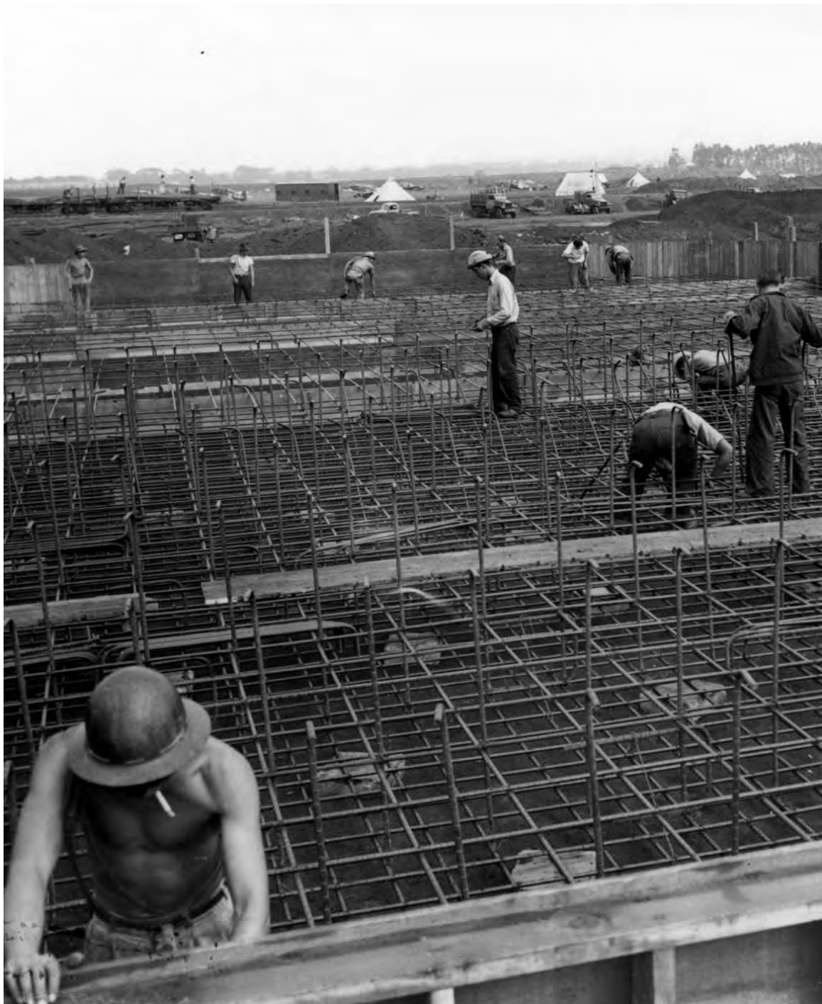
CONSTRUCTION WORK AT WHEELER FIELD, 11 December 1941. After the Japanese raid many destroyed or damaged buildings were rebuilt.
