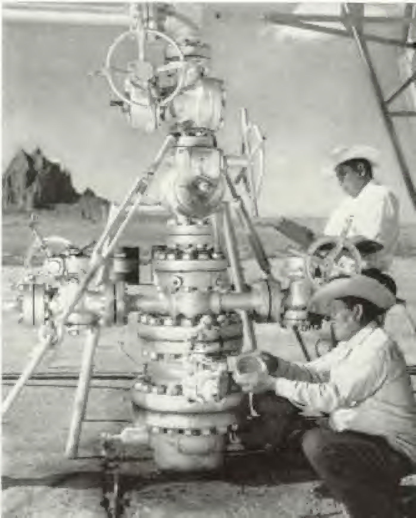
Maze of valves regulates the flow of a helium-bearing natural gas well. These Navajos check wellhead pressure below Ship Rock, a butte in New Mexico.
