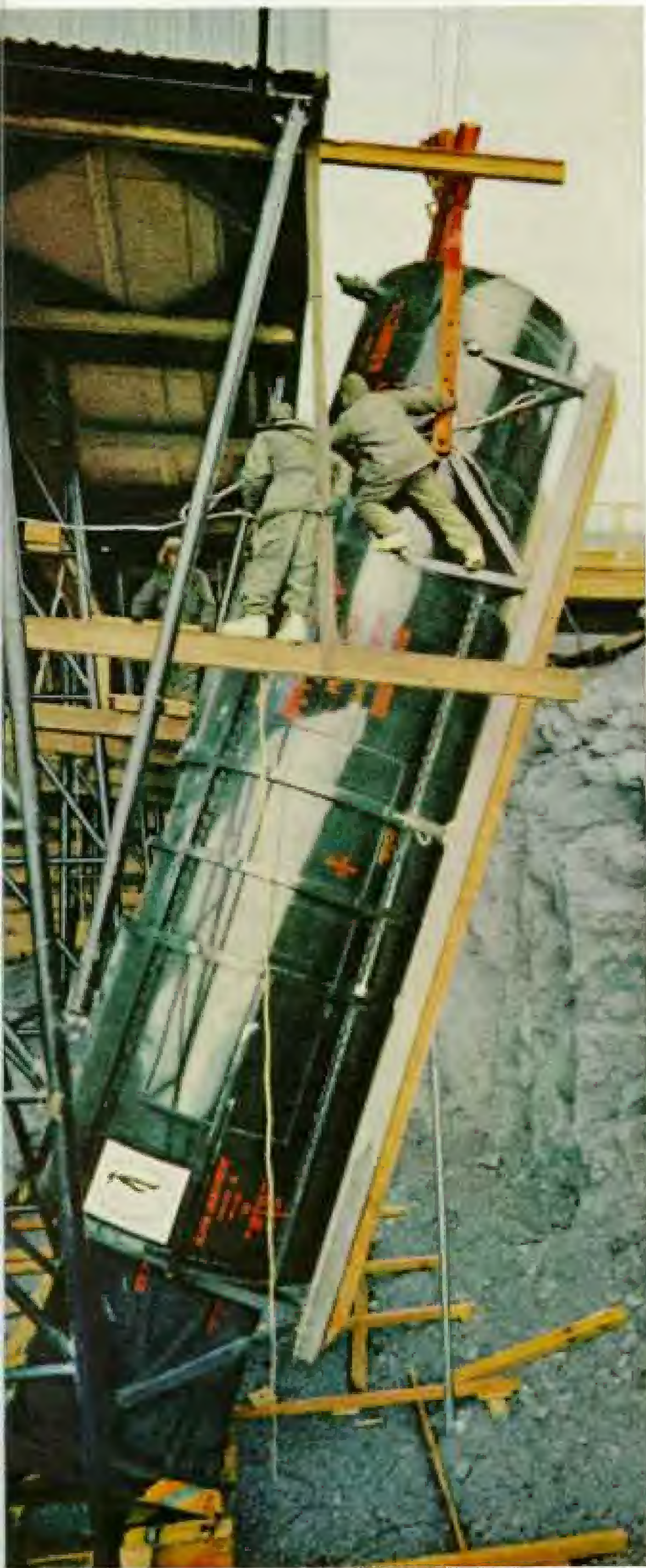
Waste processing container for McMurdo's reactor sinks into rock under the skillful guidance of Seabees.
