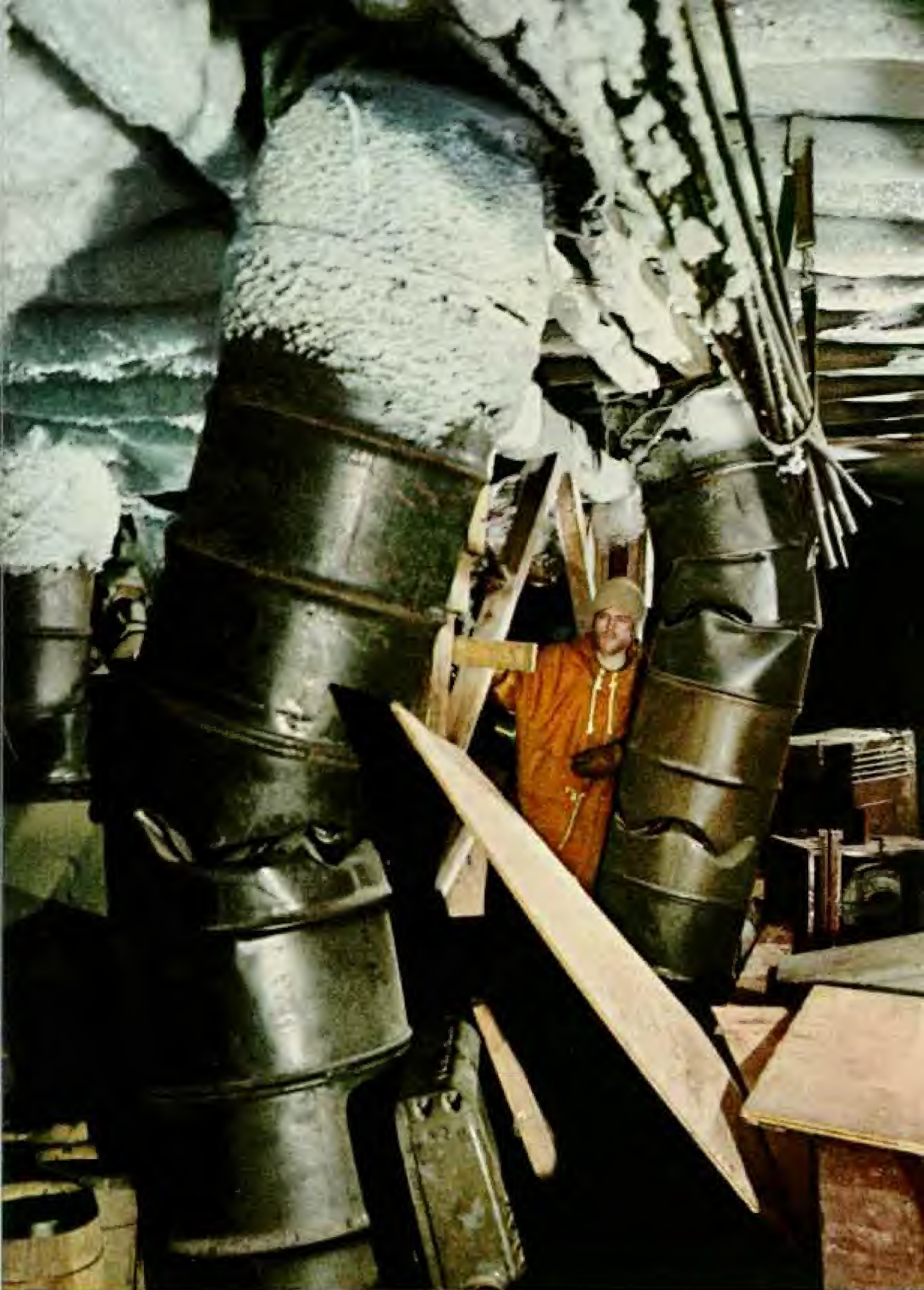
Oil-drum pillars crumple at old Byrd Station. Roof sags under tons of crushing snow
