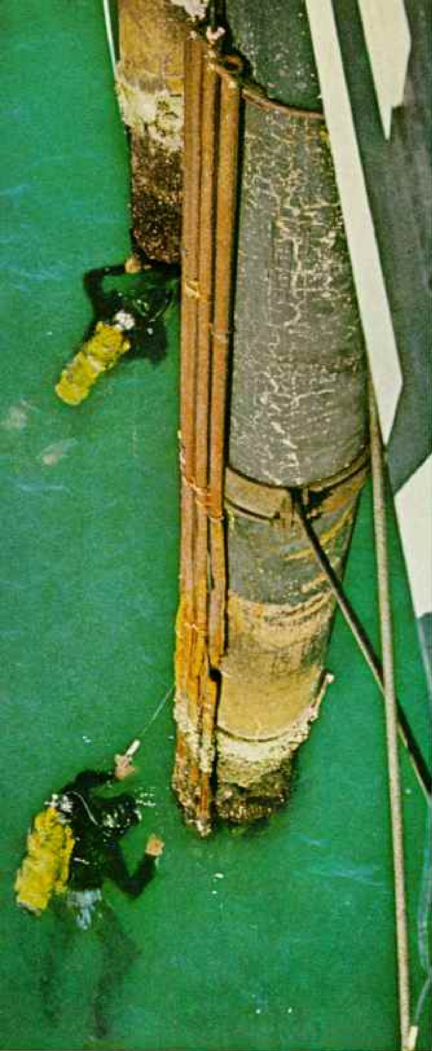
Divers hack at marine organisms growing on the piling of a pier off La Jolla, California. They seek anemones for the author to photograph (pages 268-9). Tricky swells make their work hazardous.
