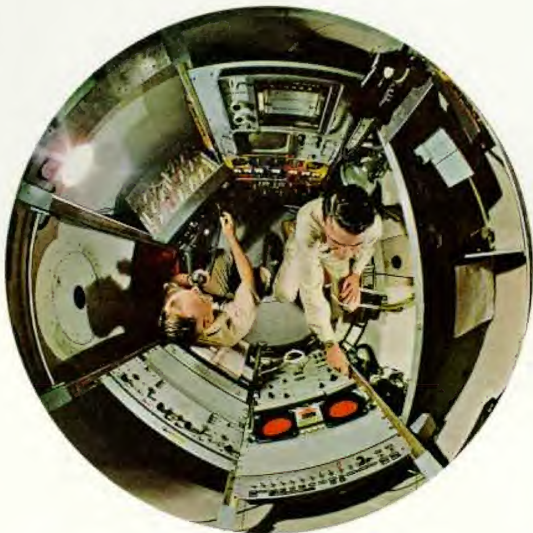
Cramped bathynauts sit hemmed in by batteries, echo sounder, gyroscope, TV, and controls. Lt. George W. Martin (left) telephones the surface; Commander Keach checks the sonar. Camera with 180-degree lens took the picture.
