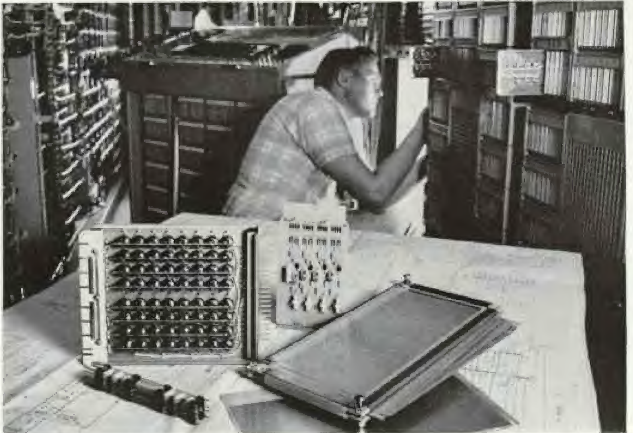
CENTRAL CONTROL SECTION that handles logic and command functions for ESS is shown in background. Foreground shows basic components.
