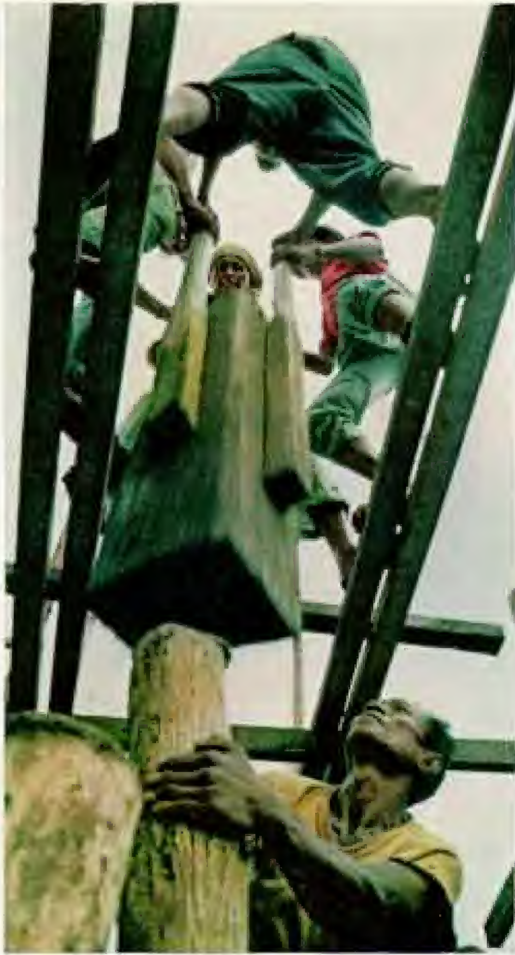
Man-powered pile driver sets wooden pilings into Jolo's tidal flats—first step in building a Moro house in the Sulu Islands. A floor, walls, and thatched roof complete a one-room dwelling. Simple furnishings include sleeping mats and earthen hearth.
