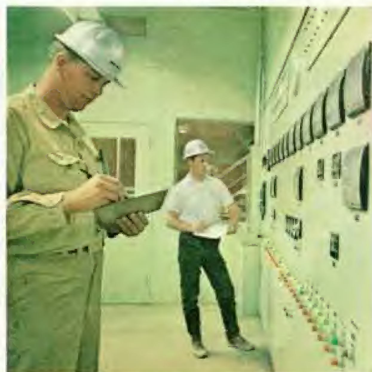
Electronic control panel monitors milling process.
