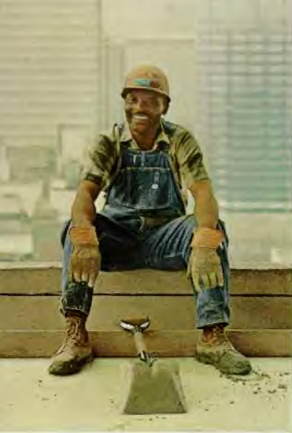
With a hand in the new Atlanta, construction man Ed Morgan works with a concrete-flooring crew high on the Trust Company of Georgia building. By attracting business, metropolitan Atlanta each year creates more than 26,000 jobs.
