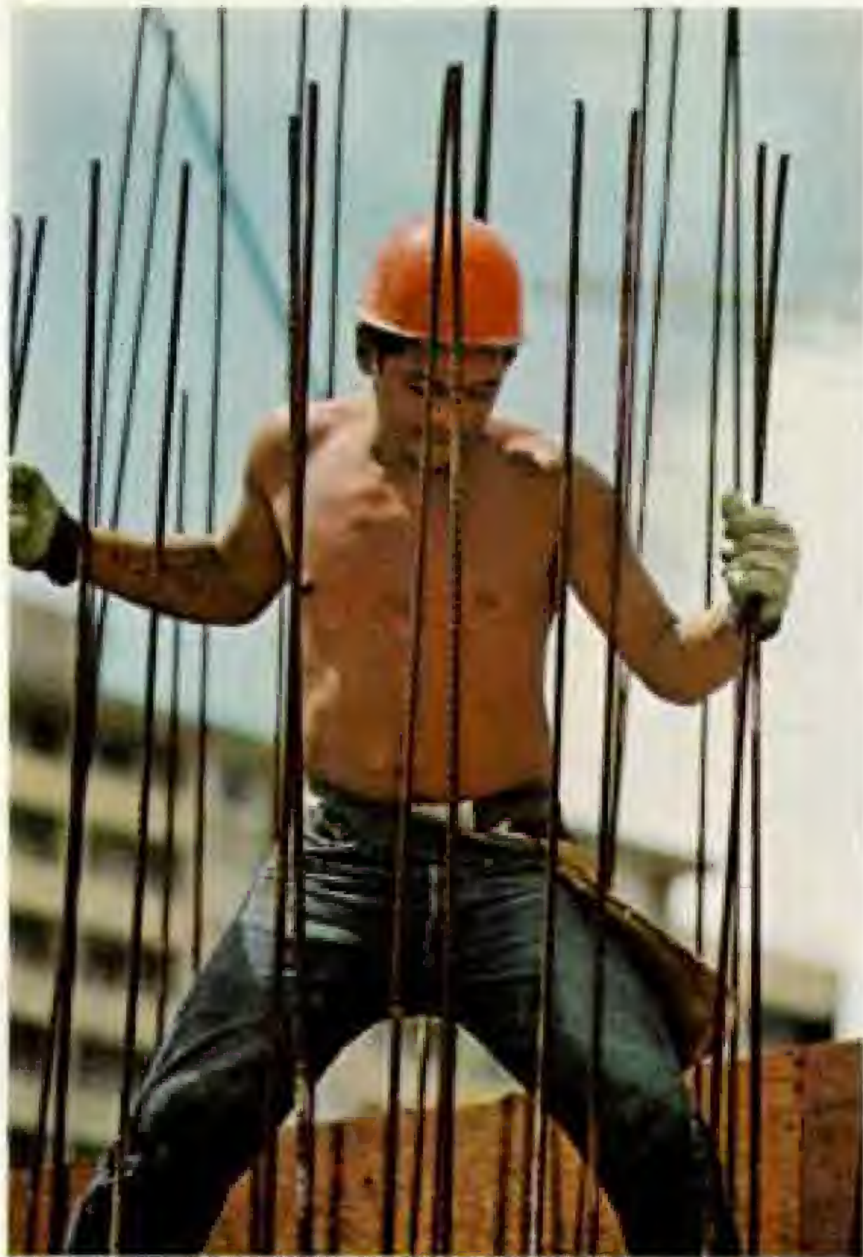
Muscle counts as a worker aligns steel reinforcing rods, a common sight in a city bustling with construction activity. Yet housing remains in short supply and may cost twice as much as on the mainland. The high cost of living reflects the expense of shipping most goods from the West Coast, 2,500 miles away.
