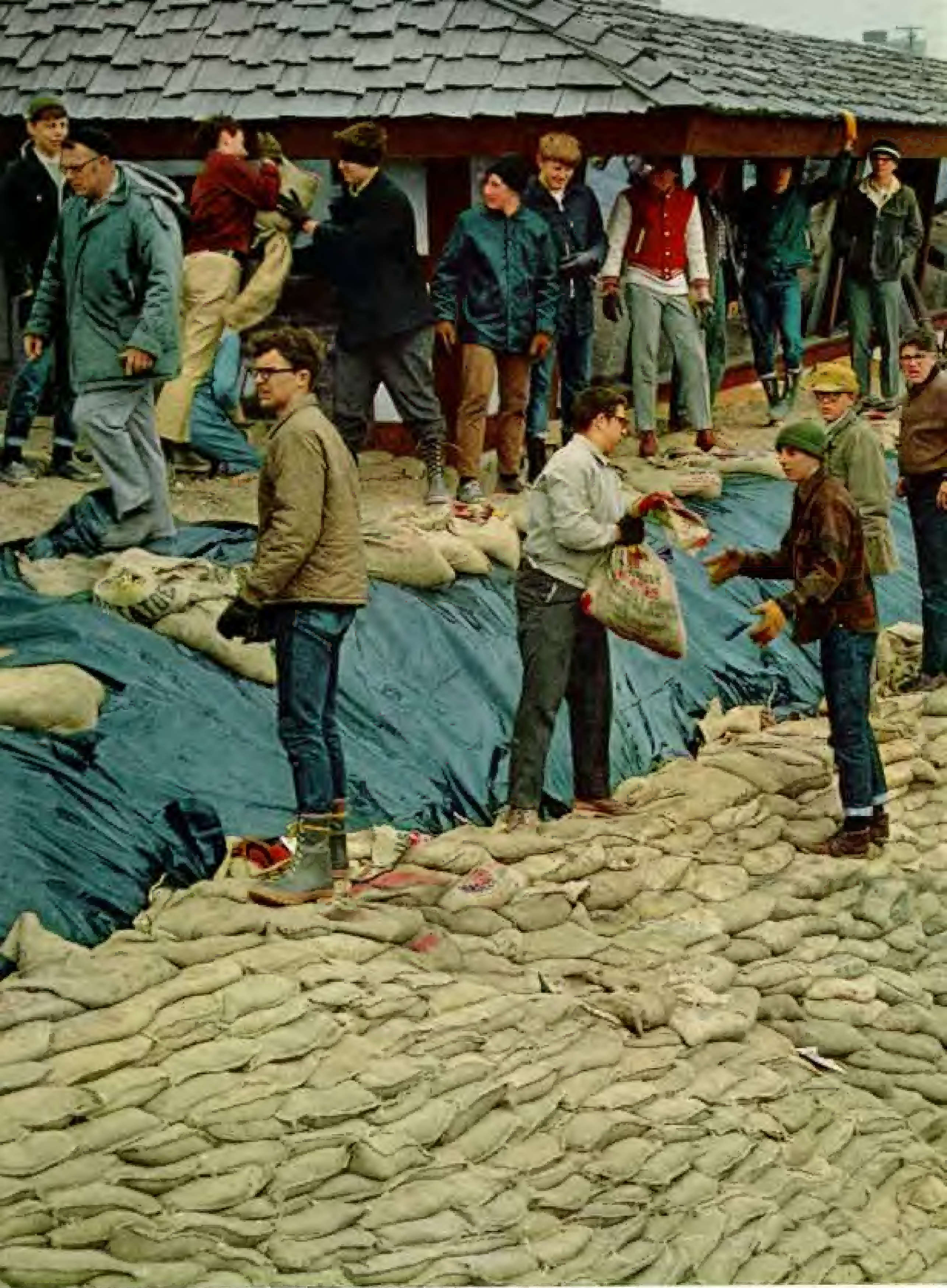
Forewarned, forearmed: A battlement climbs toward the caves of the Century Club Restaurant in North Mankato to stave off the rising Minnesota River. Sandbags anchor sheets of polyethylene plastic to prevent scouring by currents. Most of the workers are teenagers—
