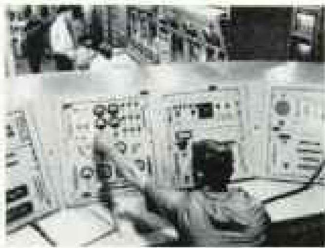
Control Room For 20-foot-diameter Starboard Antenna
