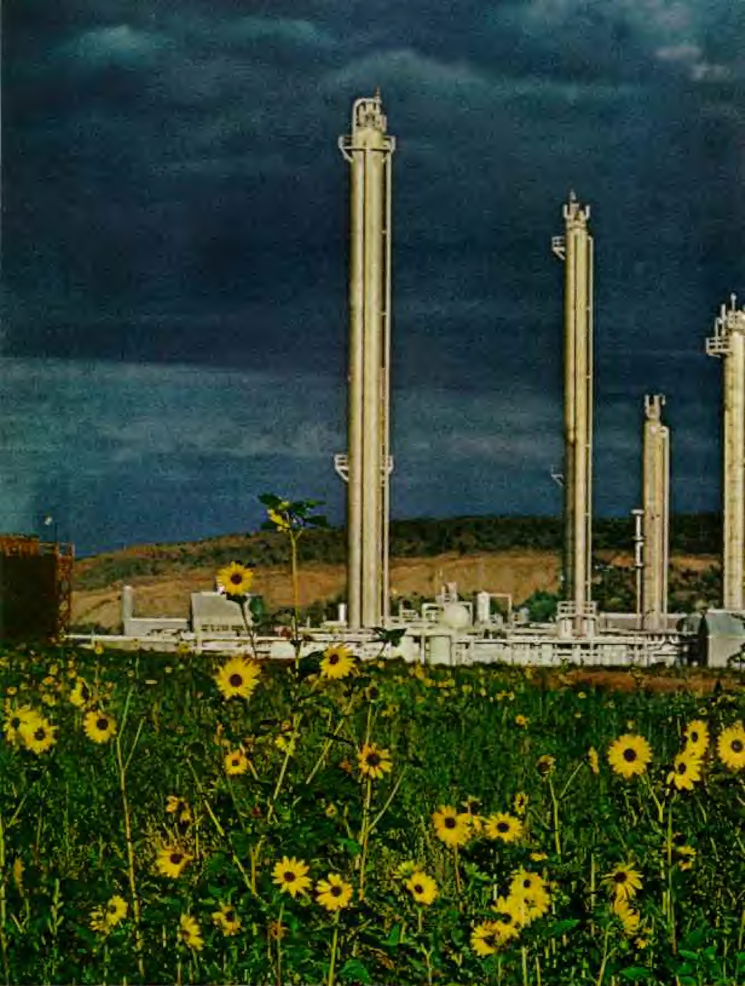
Fire and storm lend an infernal look to a coneflower-strewn field near Gallup. At the Wingate plant of El Paso Natural Gas Company, flames belch from a waste pit; in the distance rise silvery fractionating towers. Such plants of the El Paso system compress natural
