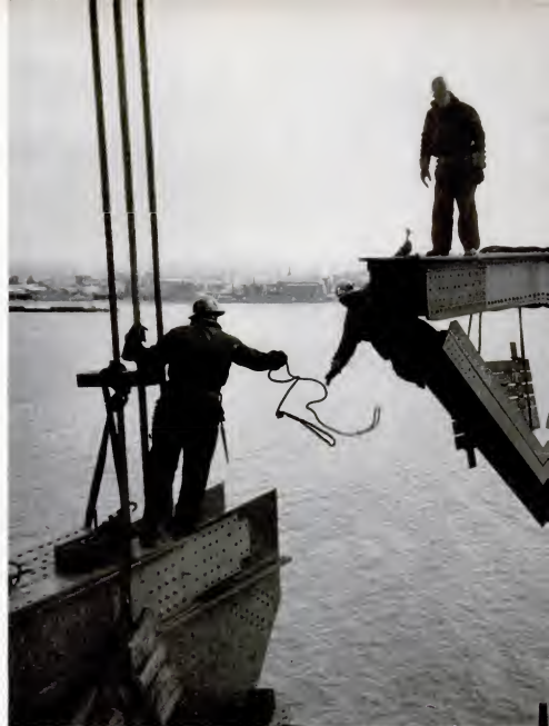
RAISING A TRUSS , men of the raising gang ride the swinging steel 100 feet above the water. They jumped on to it when the truss was swung near the
