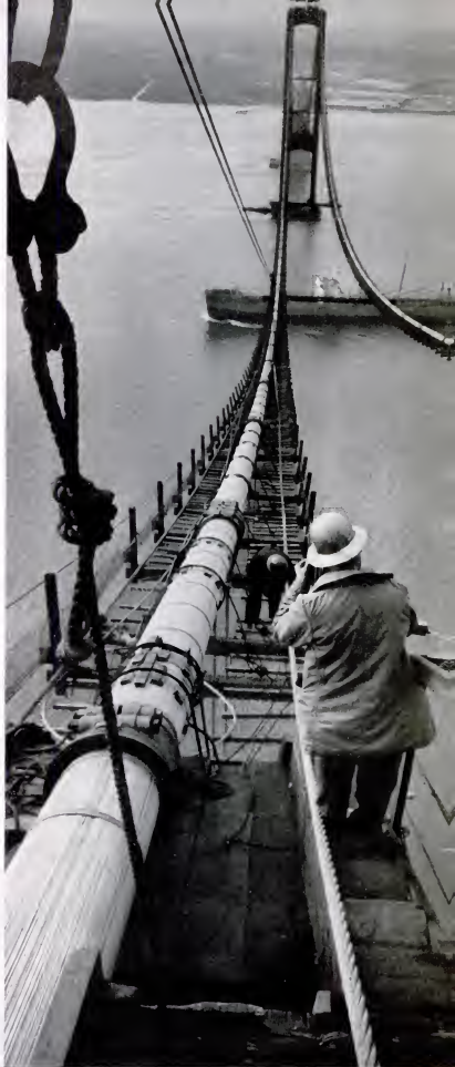
THE MAIN CABLE, which was spun strand by strand between the shores, is now bound tightly together. Later it will be wound around with galvanized wire. Then catwalk will be removed and two hand ropes will be strung along top of cable.
