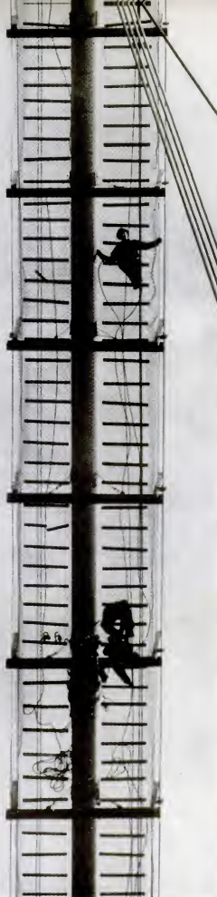
ON THE GATWALK , which was strung even before the main cable, crew reels in small cables which originally held catwalk up. These will be used again.
