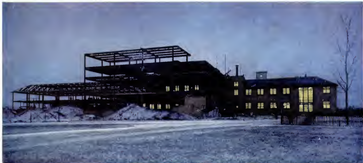
TO TRIPLE THE CAPACITY OF ITS ELECTRONICS LABORATORY at Electronics Park, near Syracuse, N.Y., General Electric speeds completion of a new laboratory wing. Lights burn late as a growing army of scientists and engineers at G.E.'s modern
