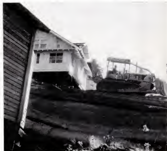
SALVAGED HOUSE is towed away intact by a bulldozer to vacant lot in less slippery part of town. →
