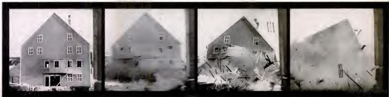
CANNING FACTORY OWNED BY A NORWEGIAN QUISLING IS WORKED ON BY BRITISH DEMOLITION EXPERTS. MOMENT OF EXPLOSION IN SECOND PICTURE SHAKES THE CAMERA
