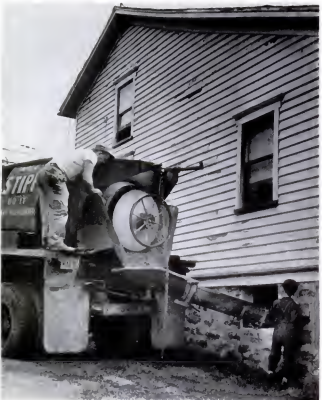
CLOSING CRACKS in the basement of a house on Cedar Avenue near the fiery mine, a truck pours concrete to seal off fumes seeping through earth.
