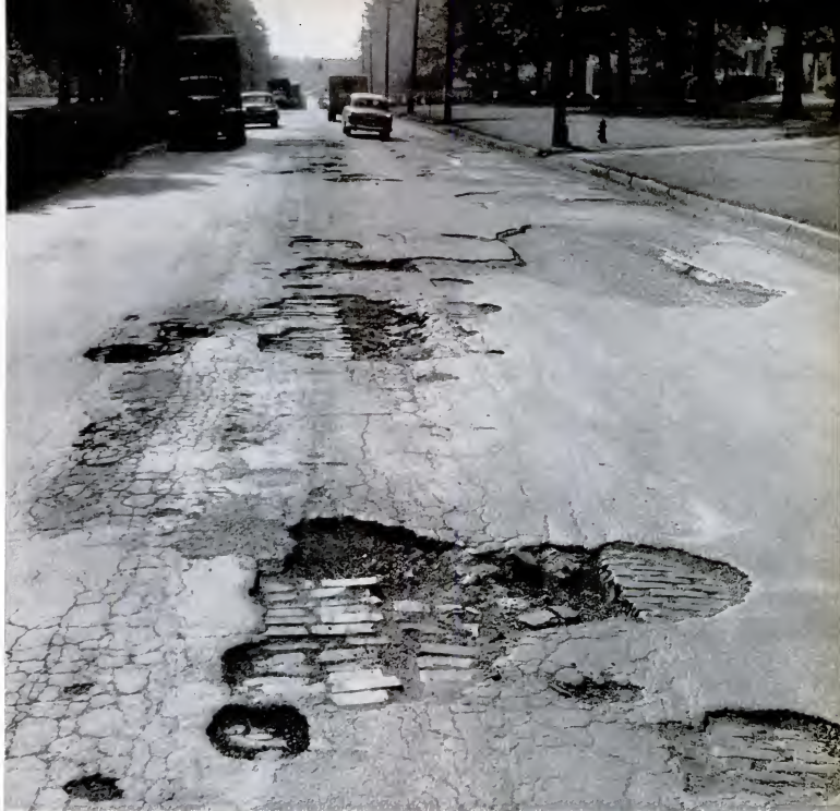
THESE DEEP, AXLE-BREAKING HOLES IN AN OHIO TOWN'S MAIN STREET (U.S. ROUTE 20) HAVE BANGED UP TRUCKS AND CARS, AND CAUSED DAMAGE SUITS
