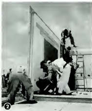
2 With one wall already up, workmen tighten its connections to frame and get ready for next one.
