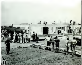
3 Hearty heave gets "white" end wall in place, leaving "blues" far behind. Workmen from other houses knocked off to watch.
