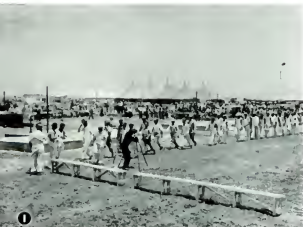
1 Skilled 50-man building team files to position beside prepared foundation. Pre-fabricated sections were assembled under tents at the rear.
