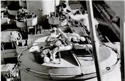
REMOVING LID of one of the ship's two stacks, work detail detaches the pipes connected to the dehumidifying
