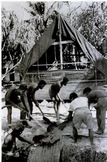
ON RONGERIK , their new home, industrious natives and Seabees mix cement to make cisterns to catch rain. There is no water on any of these small atolls in Marshalls.
