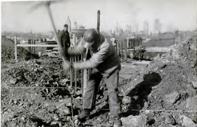
WORKMEN DIG FOUNDATIONS FOR A NEW HALLMARK GREETING CARD PLANT TO GO UP WITHIN THE CITY LIMITS OF KANSAS CITY, WHOSE SKYSCRAPERS RISE IN THE DISTANCE
