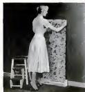
EASY. Slowly unroll strip and apply to wall. No need to hurry... adhesive stays moist for more than 15 minutes.
