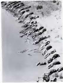
ALONG BANKS, chains of old cars serve as revetment to prevent swirling water from eroding soil.
