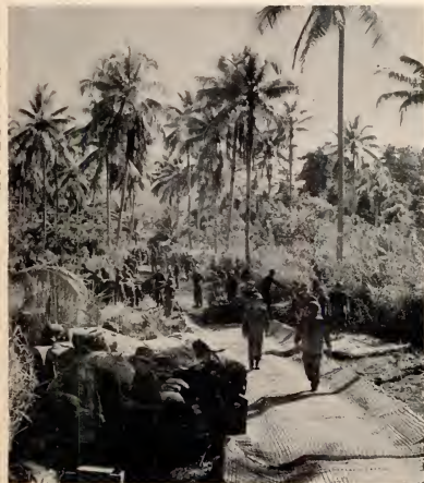
Road to Lao is covered with steel mats by U. S. Engineers as the attack progresses. Japs, who could see it in the jungle, made a point of flying low and strafing men working on it. These nuisance raids only interrupted progress for a time, the Engineers went right back and soon had the job completed.
