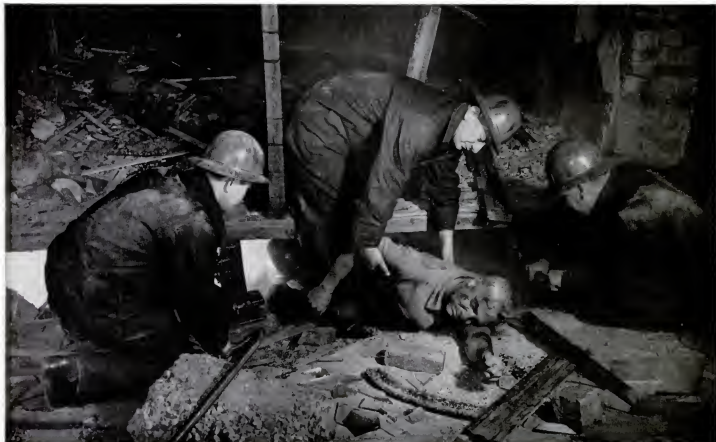
Victim is extricated, in a police rescue demonstration, from cellar of partly demolished building. Fifteen-ton jacks have
